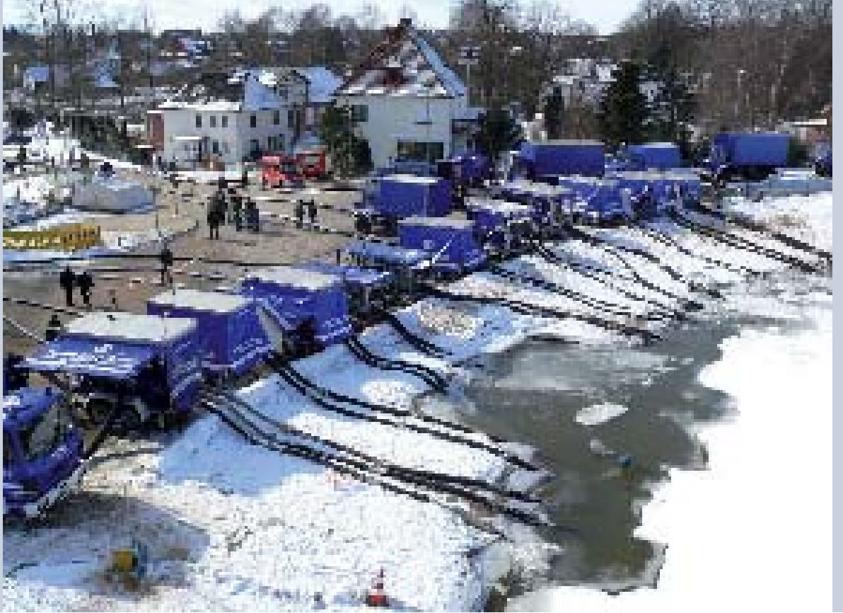
Pressure from melt water threatens to break a barrage. Source: German Federal Agency for Technical Relief (THW)
